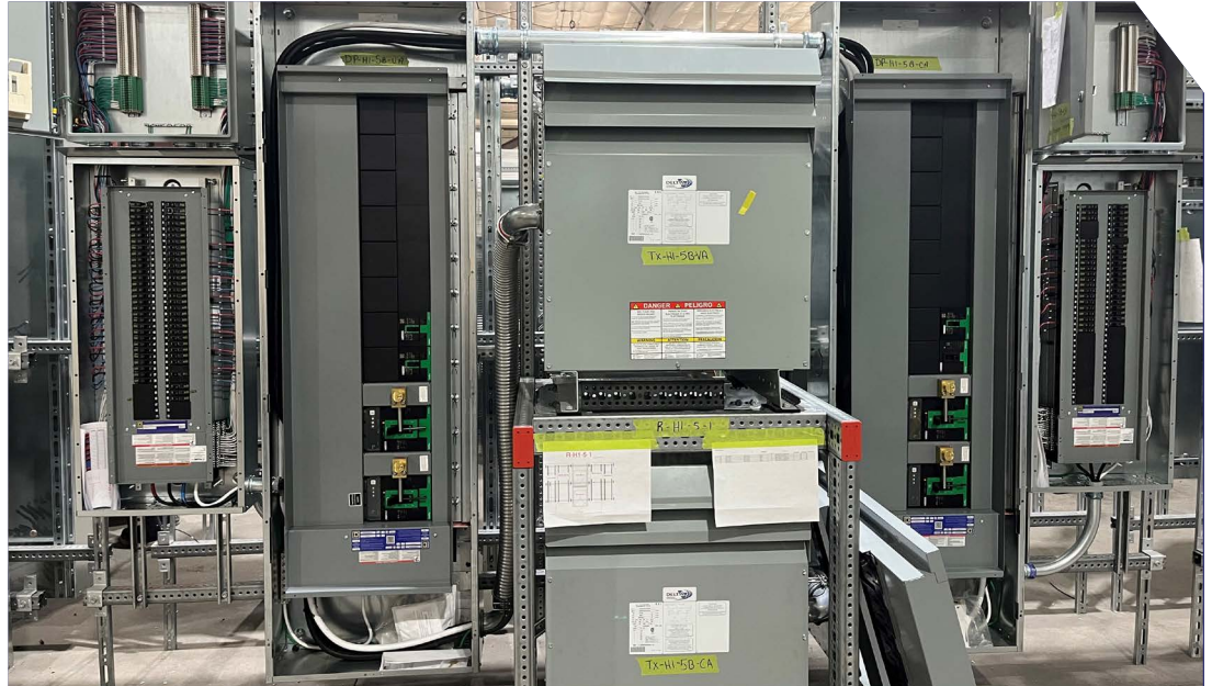
→ Electrical racks like this will power the hospital.
